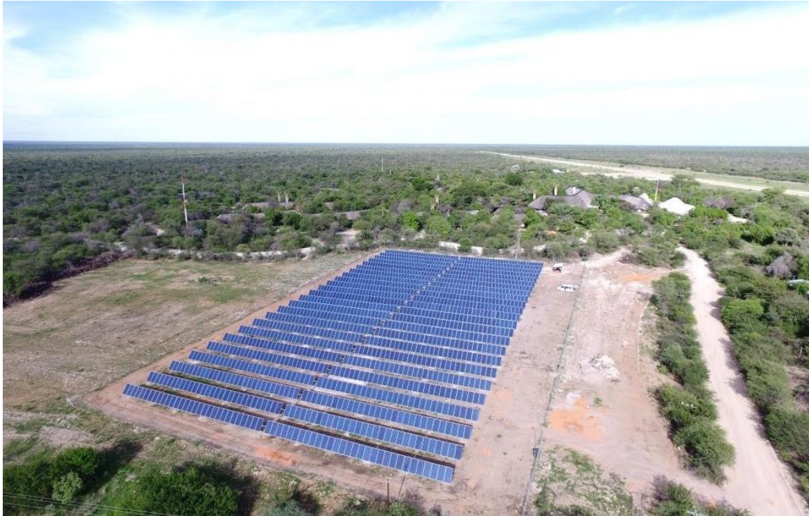
Solar Plant at Mokuti Etosha Lodge, Namibia.
